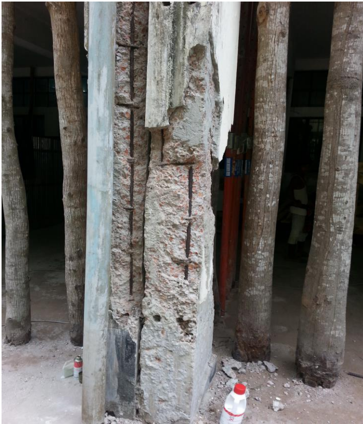
Fig: Dilapidated columns
